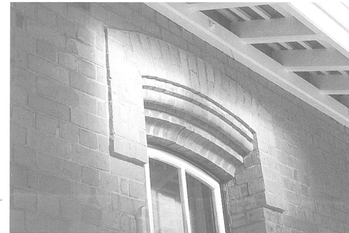
BELOW: Details of purpose-made replicated brickwork. Voussoir bricks to the hood; and the segmental arch composite of both roll and gorge moulded bricks.
